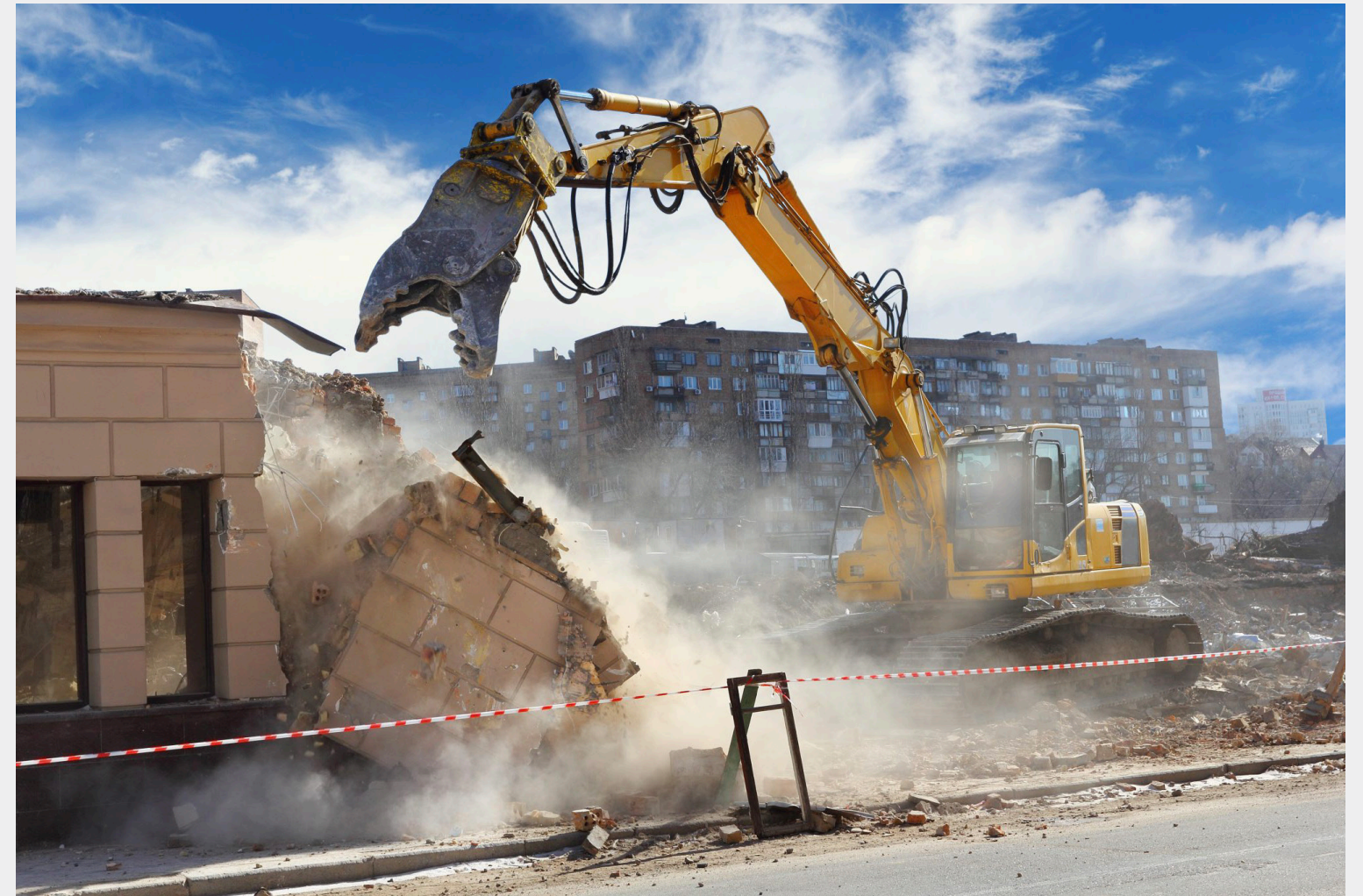
Image: Unplanned, unstructured, and unregulated conventional demolition practices result in negative environmental impacts, including risks to public safety. The recycling rate of demolition waste in such cases remains very low [11].
