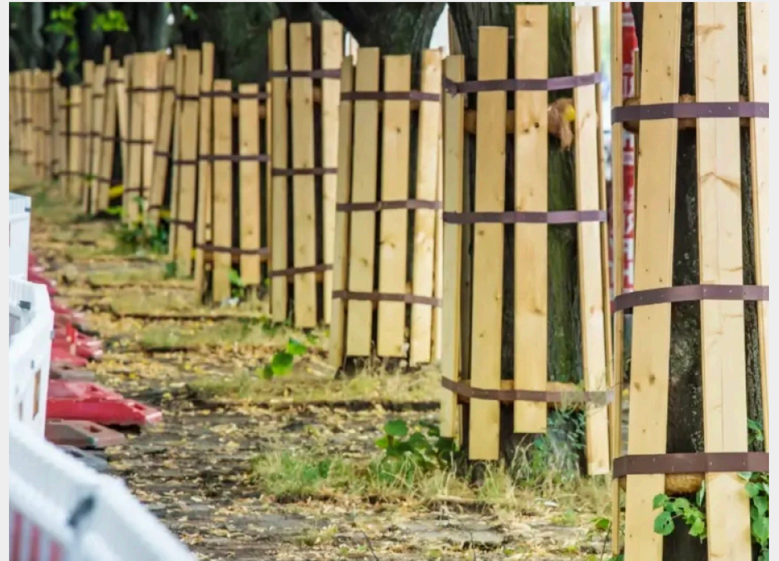
Image: Existing trees in the construction area should be protected from heavy machinery impact using protective barriers and equipment [19].
