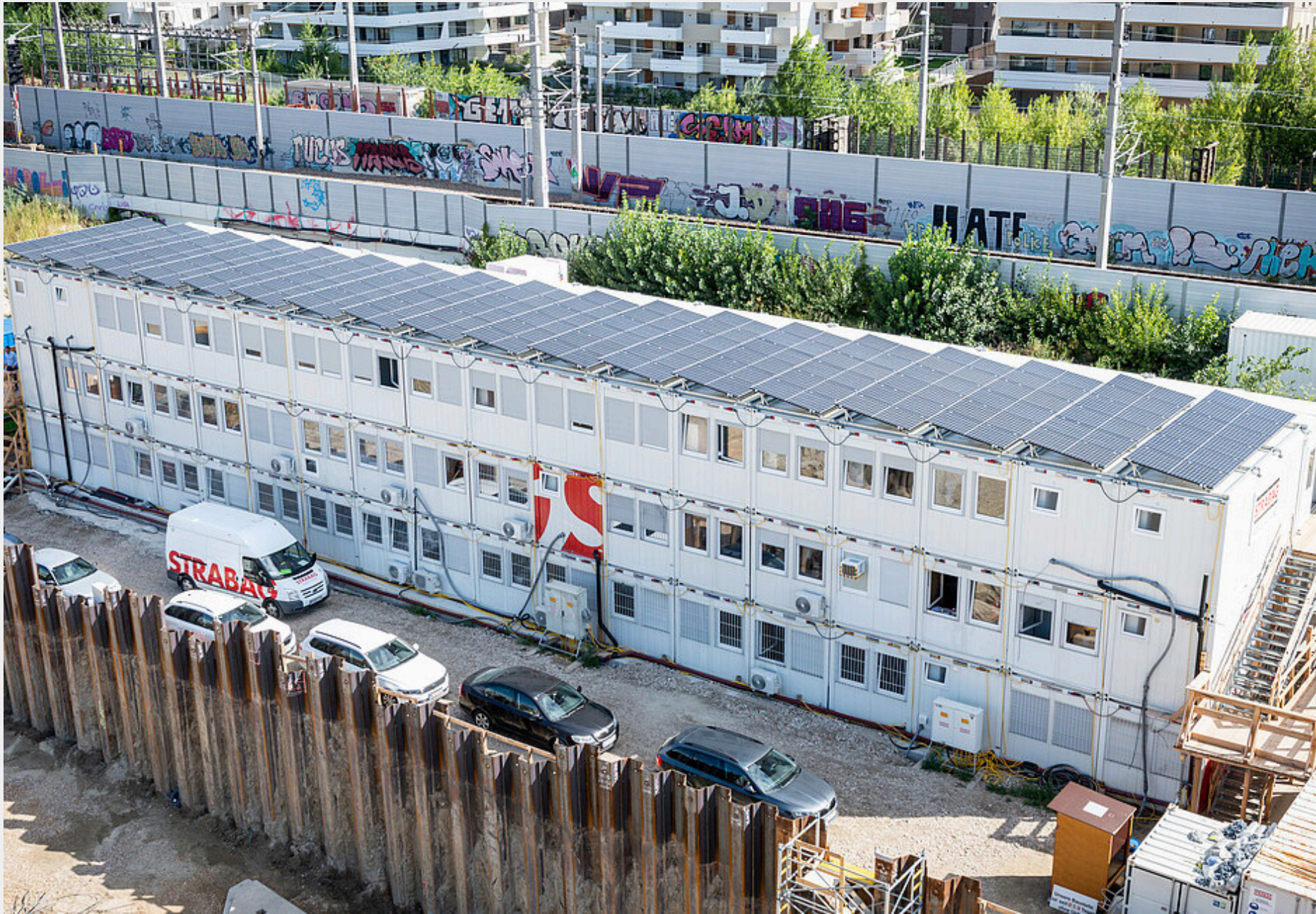
Image: Passengers traveling by train in Vienna can see the first photovoltaic system installed on the roof of the temporary construction site office of the Northern Railway Station construction project when looking out the window between Praterstern and Traisenstraße stations. This is an example of a construction project that meets its own energy consumption through PV panels [3].
