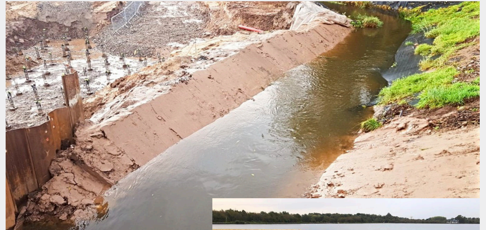
Image: The negative impact of construction on nearby water resources [22].
