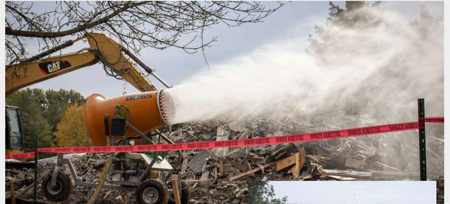
Visual: Dust suppression system with water spraying [44].
