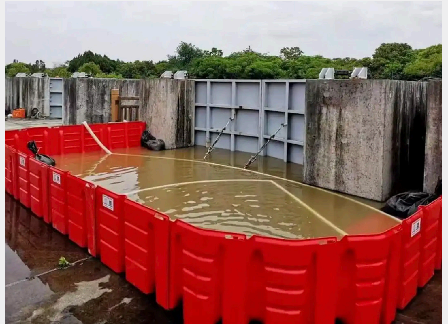
Image: Temporary barriers to prevent flooding from urban flooding impact at the construction site. These barriers help prevent loss of life, property damage, and pollution [28].
