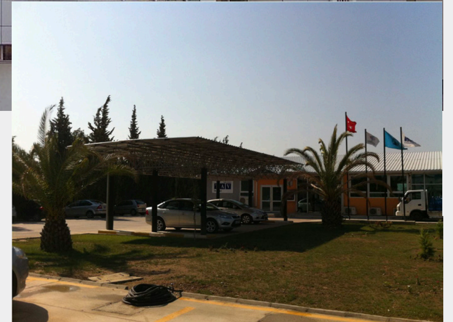
Image: The construction site buildings, parking lot shading elements, and all permanent construction site structures of the Izmir Adnan Menderes Airport Domestic Terminal were built entirely using salvaged building materials from the old airport structure [13].
