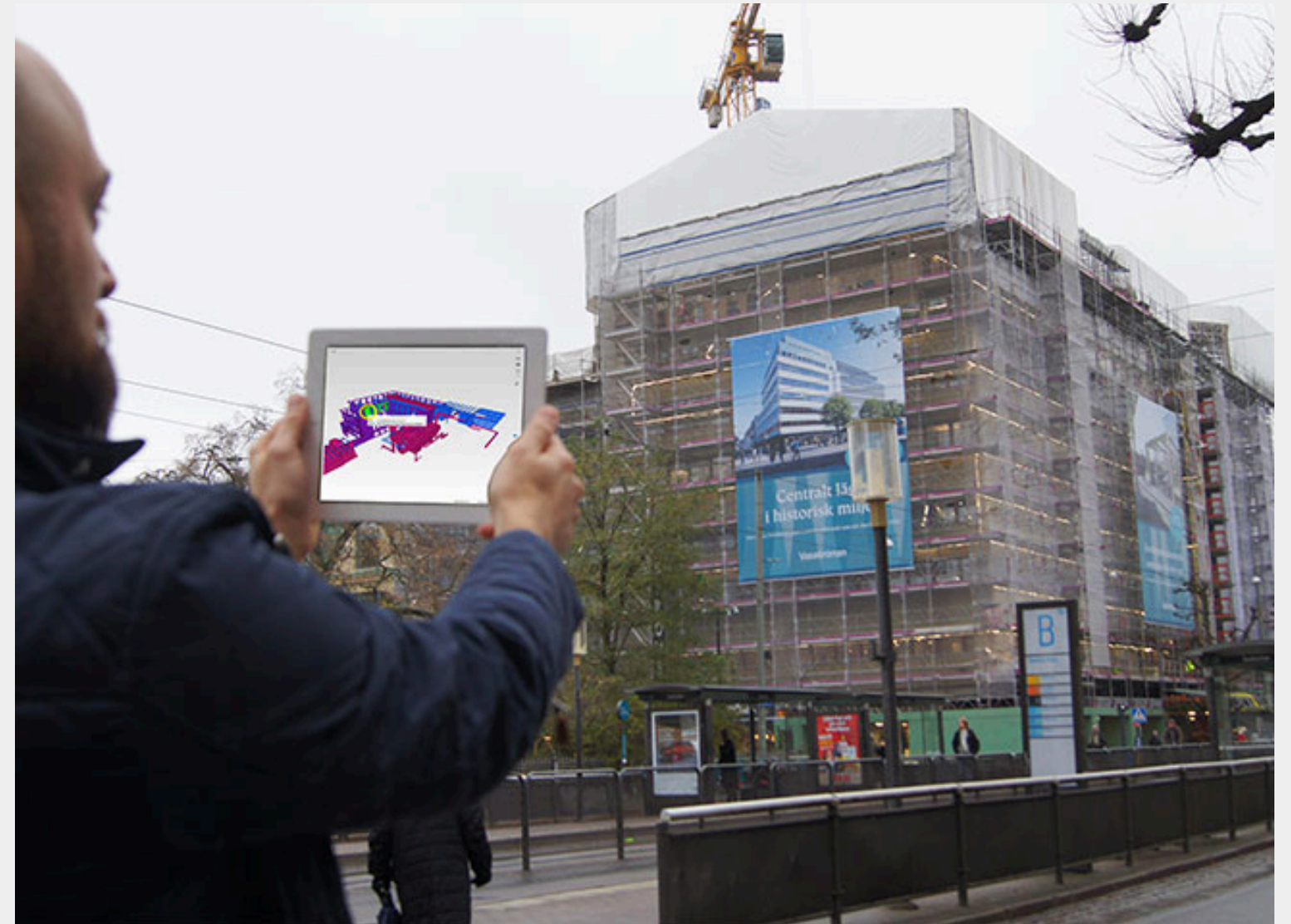
Image: A value-focused visualization based on the carbon footprint generated throughout the whole life-cycle of the Ströms building in Gothenburg. Building information system tools are used to identify the circularity aspects of the building, such as reuse, recycling, and revaluation potential [30].
