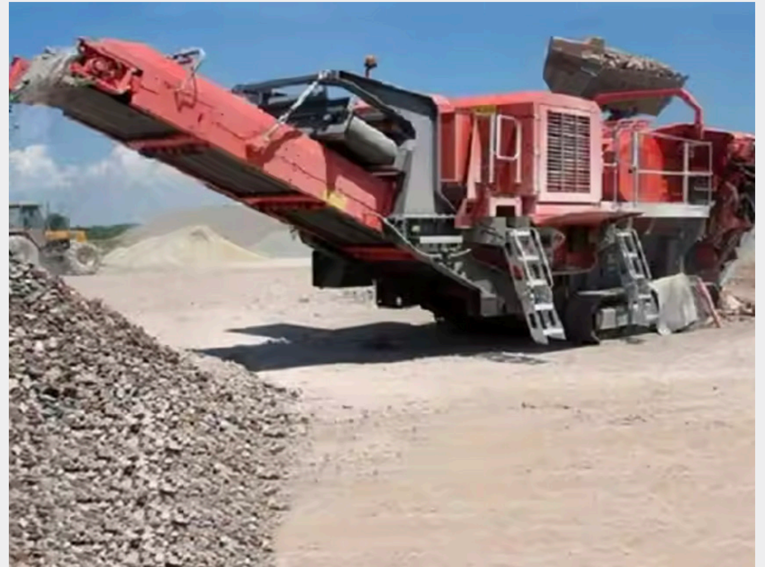
Image: Concrete fragments obtained from demolition are processed on-site using a mobile crusher and reused [18].
