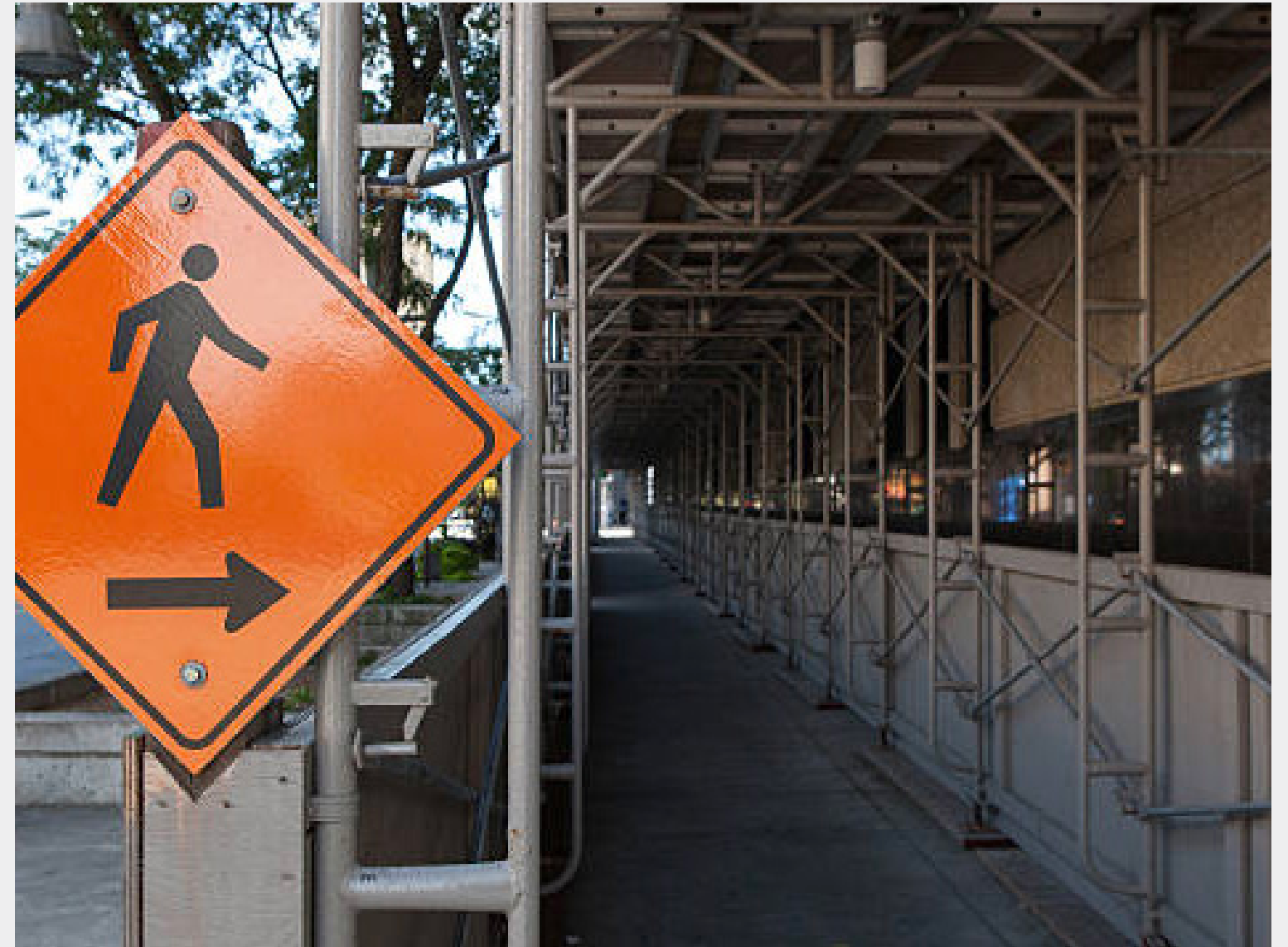
Image: Application of safe passageways and security signs around the construction site [29].
