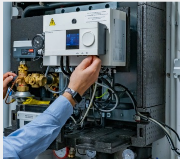
District heating building connection station © Danfoss
