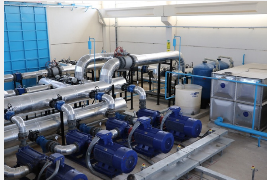
Soma District Heating System Pump Station
