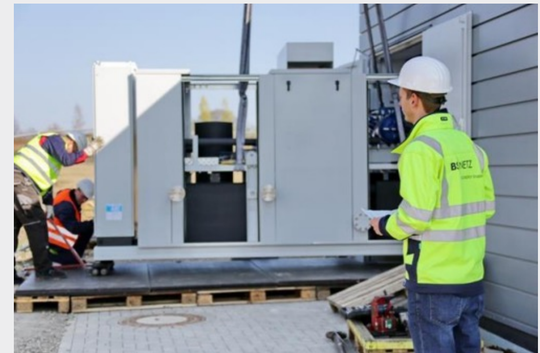
Brunswick District Heating Project Heat Pump Installation @ ReUseHeat [28]
