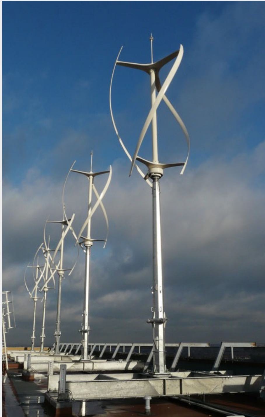
Building-Integrated Wind Turbines
