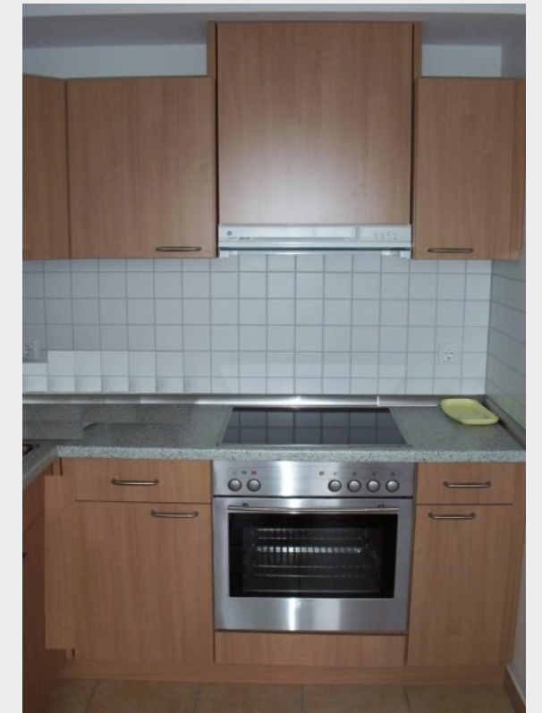
HRV unit installed inside a kitchen cabinet
