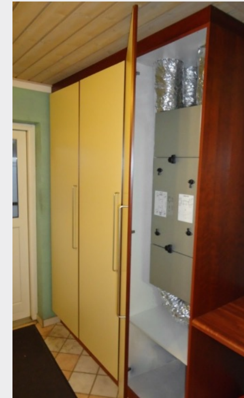
HRV unit installed inside a wardrobe
