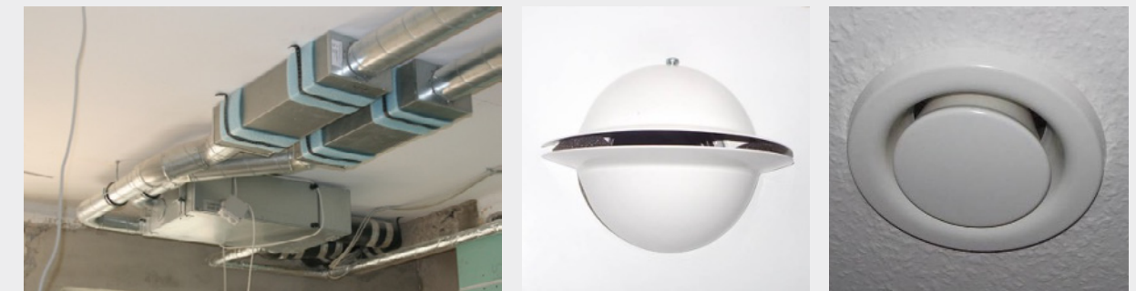
Examples of supply and extract air nozzles attached to duct terminals
